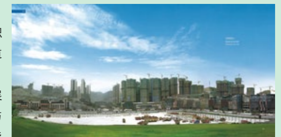
未来方舟绿色施工现场 Green Construction Spot of Future Ark Project
